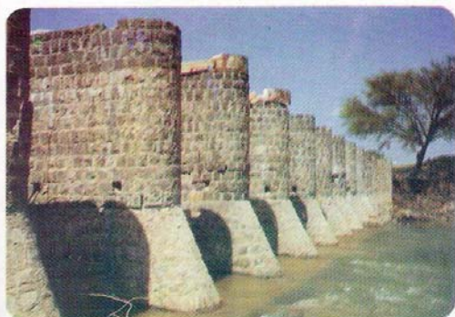
Figure 20. Hydraulic control structure near Rajegaon.
