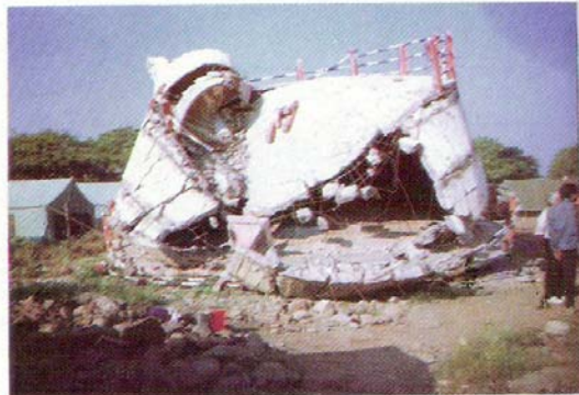
Figure 16. Circular water tank at Kavatha.
