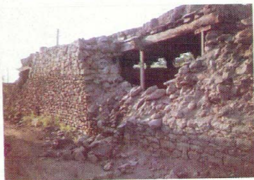
Figure 5. Khilari; Type A structure, grade 4 damage.
