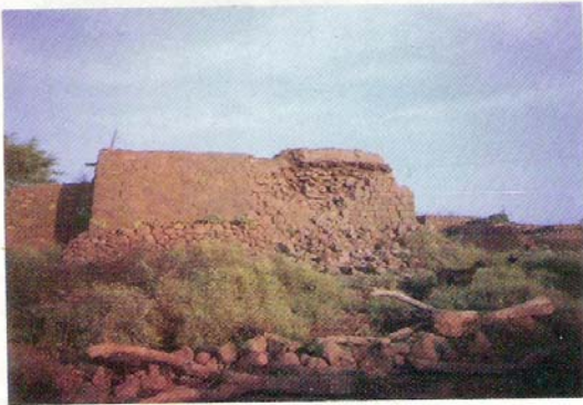
Figure 15. Bhosga-K; Type A structure, grade 3 damage.
