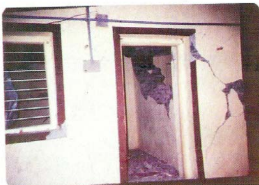
Figure 8. Khilari; Type C structure, grade 3 damage.
