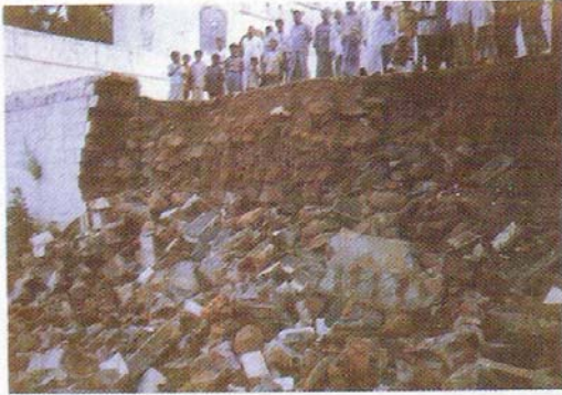
Figure 18. Retaining wall failure at Kohinoor Pahad near Basavakalyan, Bidar district.
