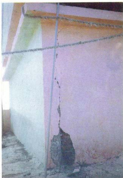
Figure 11. Umarga; Type C structure, grade 1 damage.
