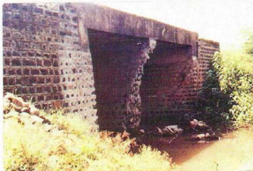
Figure 19. Damaged pier of Rudrawadi culvert near Aland, Gulbarga district.
