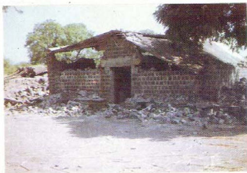
Figure 6. Rajegaon; Type B structure, grade 4 damage.
