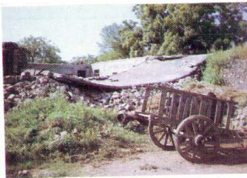
Figure 7. Kavatha; Type B structure, grade 4 damage.
