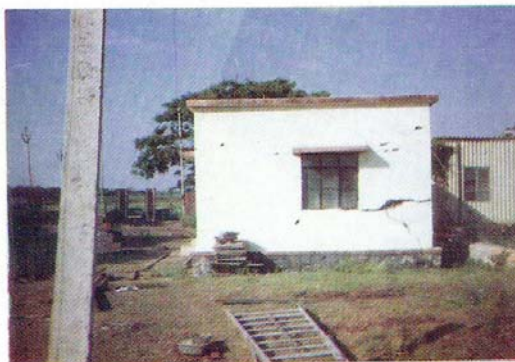
Figure 9. Sastur; Type C structure, grade 3 damage.
