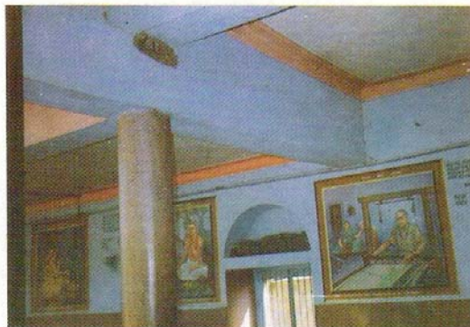
Figure 12. Basavakalyan; Type C structure, grade 1 damage.
