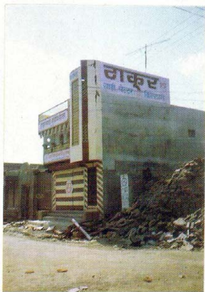
Figure 10. Khilari; Type C structure, grade 2 damage.
