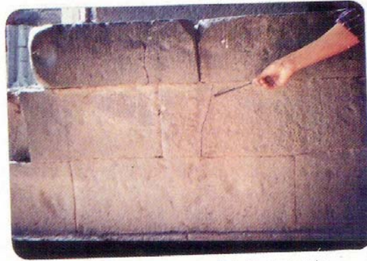
Figure 25. Cracked stone wall in Kavatha temple.
