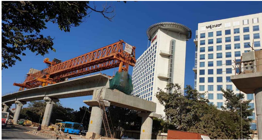
Metro extension to Whitefield has been delayed for years | Photo courtesy: Rasheed kappan
