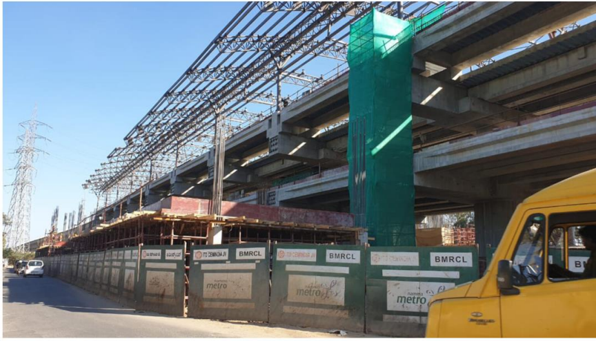
A section of the Metro extension to ITPL, Whitefield | Photo courtesy: Rasheed kappan
