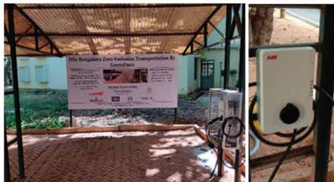
The zero emission EV charging point set up on IISc campus
